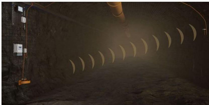
Figure 3. The Vigilante AQS is a multi-variable IIoT device monitoring air quality and quantity. Blast gas levels are monitored, allowing for a quicker and safer return to the face.
